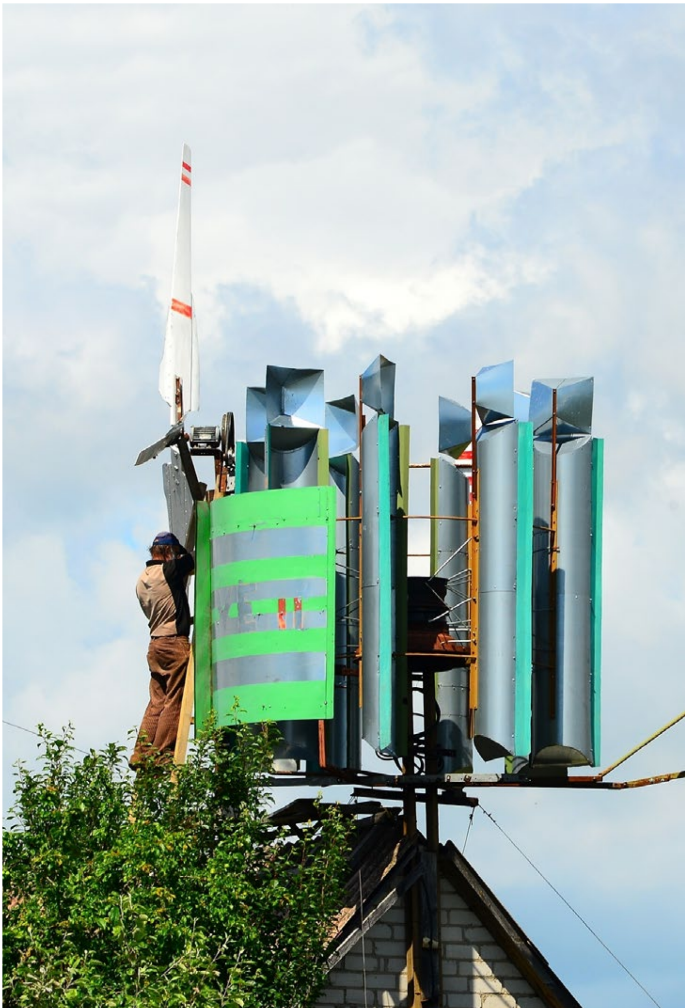
Wind electricity generator on a house roof in Seredzius town on June 27, 2015, Seredzius, Lithuania.
